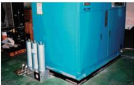
Lubricating oil for the 75 kw screw compressor (SRC-813-C)
