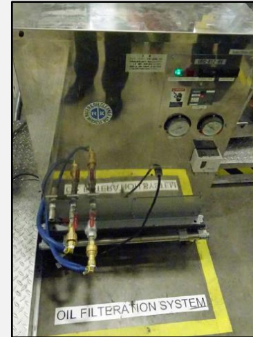
MB SRC-812-6V is installed
