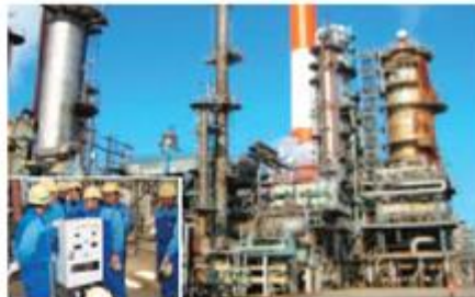
Refinery turbine lubricating oil (SRC-814-15V; explosion proof)
