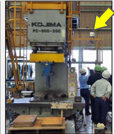
Installed in 300t press
